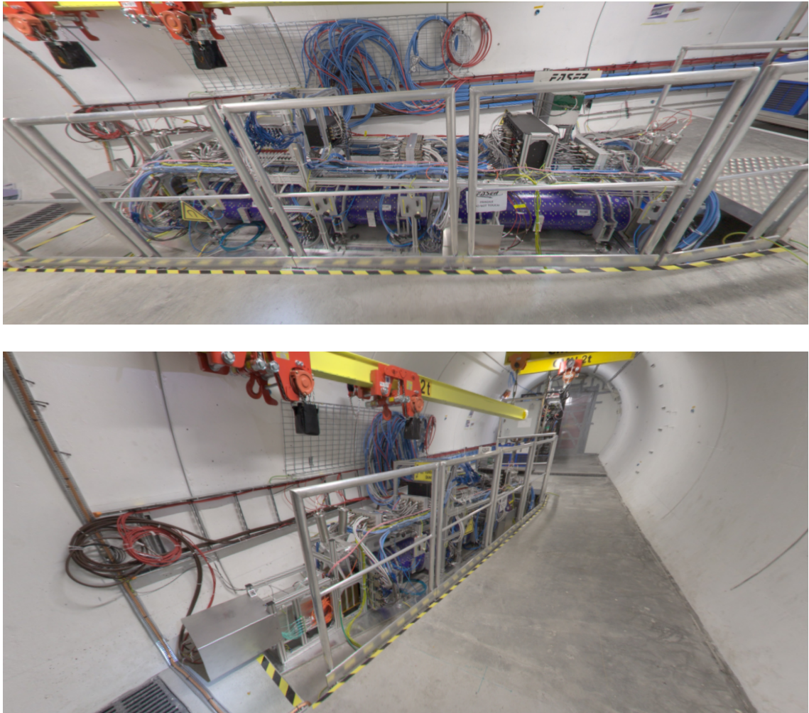
Figure 6.4: Location of FASER in the TI12 tunnel (top) and detail of the detector (bottom) before the start of Run 3.
