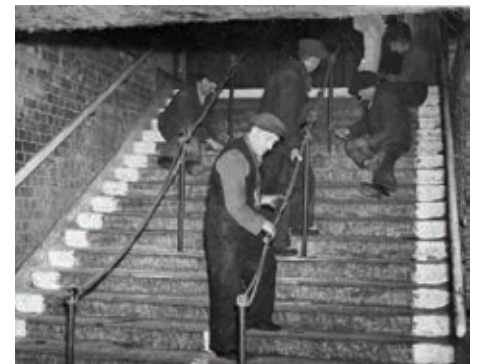
Installing handrails after the tragedy. Photo: Tower Hamlets Local History Library and Archives
