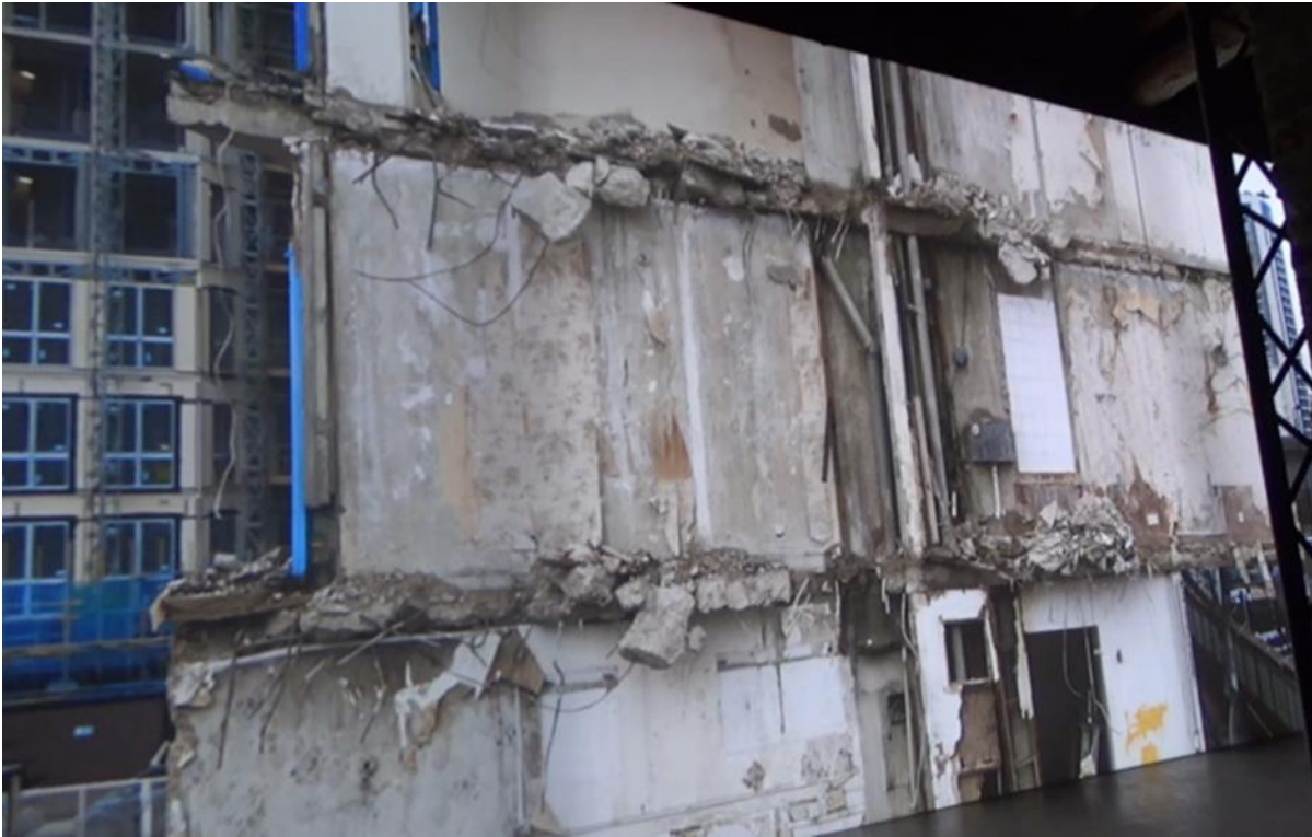
Figure 86. Still image from Do Ho Suh's video Installation at the 2018 Venice Biennale. The film pans across the west block whilst it is slowly taken apart. In the background you can see the concrete frame of part of the Blackwall Reach development also being constructed. Image taken by author (2018).
