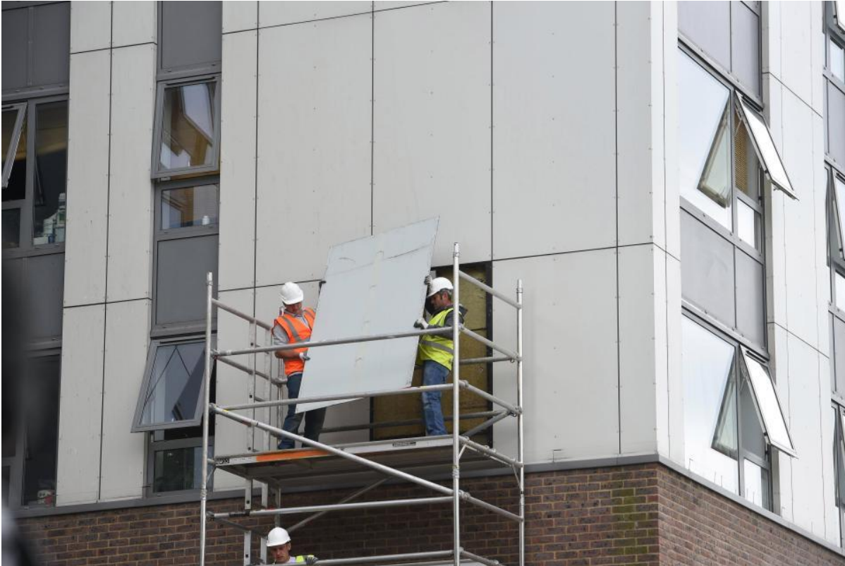
Workers removing cladding blocks similar to the ones used in Grenfell Towers
