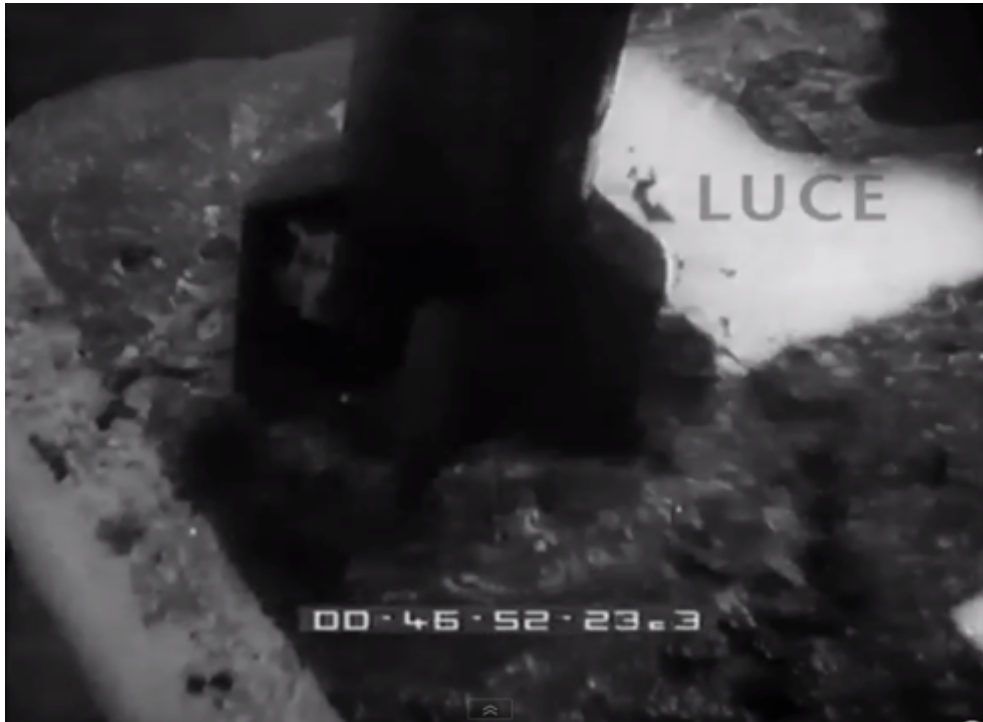
Fig. 53: The impressive force of the auger while drilling the ground, from La vita della popolazione , 18 th November 1937, Archive of the Luce Institute, Rome, consulted on 13 th May 2014.
