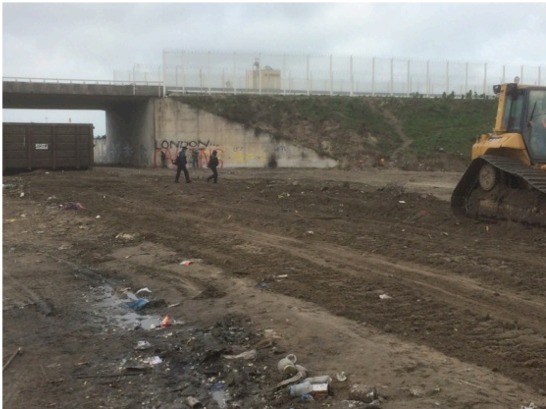
Figure 4: The construction of the 'buffer zone' between the camp and the motorway (source: author's photo)
