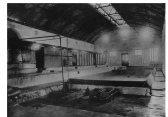
'Filtering table and boilers'
