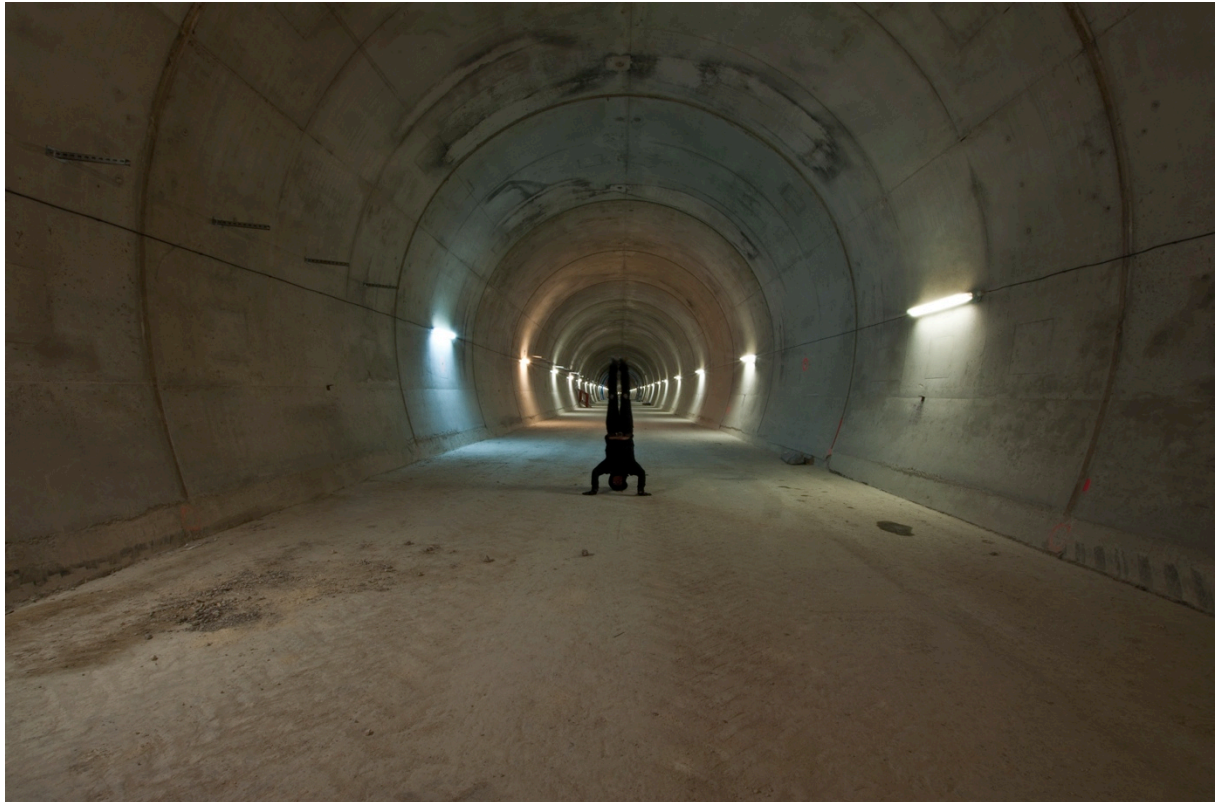
Figure 145. The author in a Metro line extension before tracks are laid, Paris, photo by author and Otter
